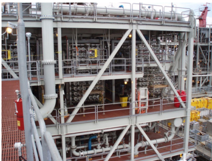
Figure 1: Sulfate Removal Membranes
