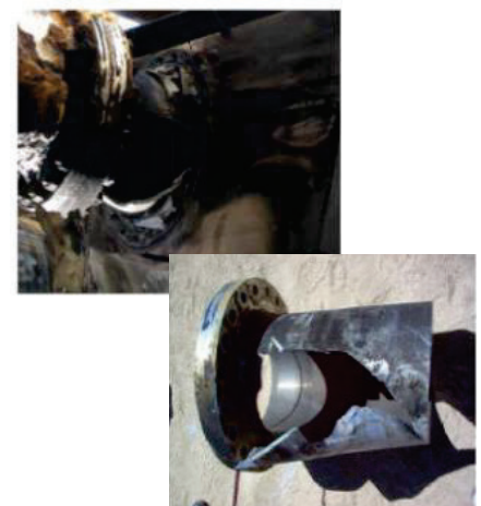
Figure 1: Moomba Gas Plant – Failed Inlet Nozzle 3
