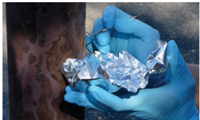
Figure 2. Corrosion debris can be safely collected for shipment in things like aluminum foil or plastic bags or plastic cups.
