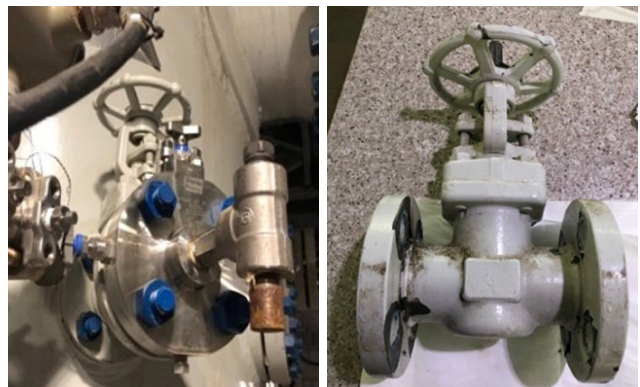
Figure 1. Seeing how the leaking valve was installed in service helped show orientation and how it acted as a suspended load. The leak was due to fatigue.
