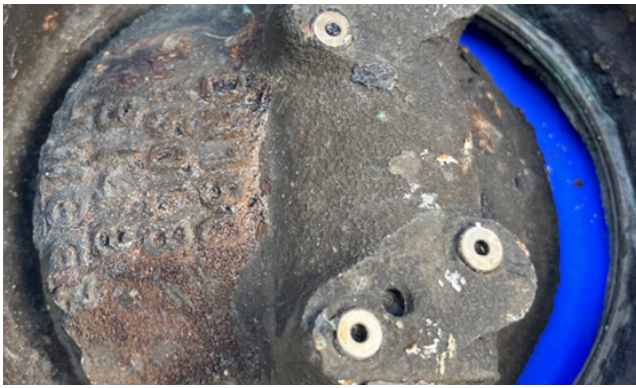
Degraded Butterfly Valve Sent in for Failure Analysis
