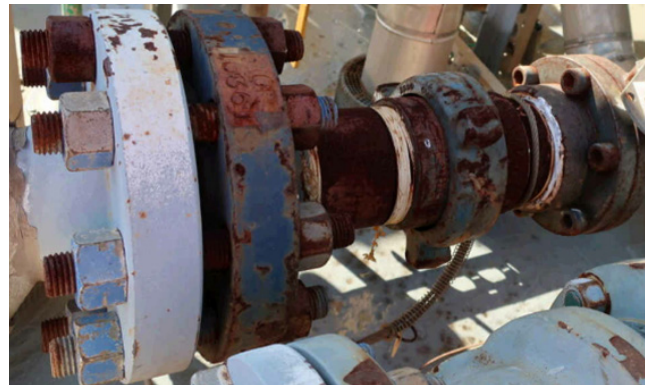
Rapid Atmospheric Corrosion on an Offshore GOM Piping Spool
